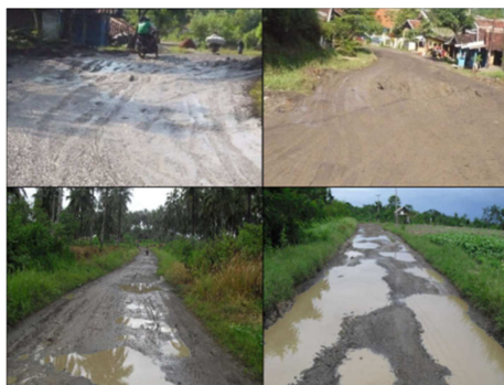
Figure 2. The condition of existing roads in the southern part of West Java before hardening with CTB.
